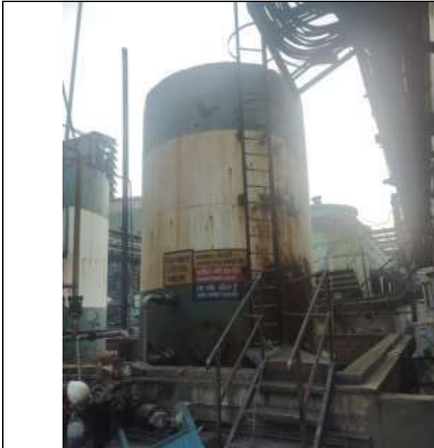
Tank in which incident occurred
