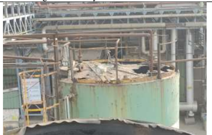
Top of the SD feed tank No-2 located adjacent to tank-1 is corroded and broken.
